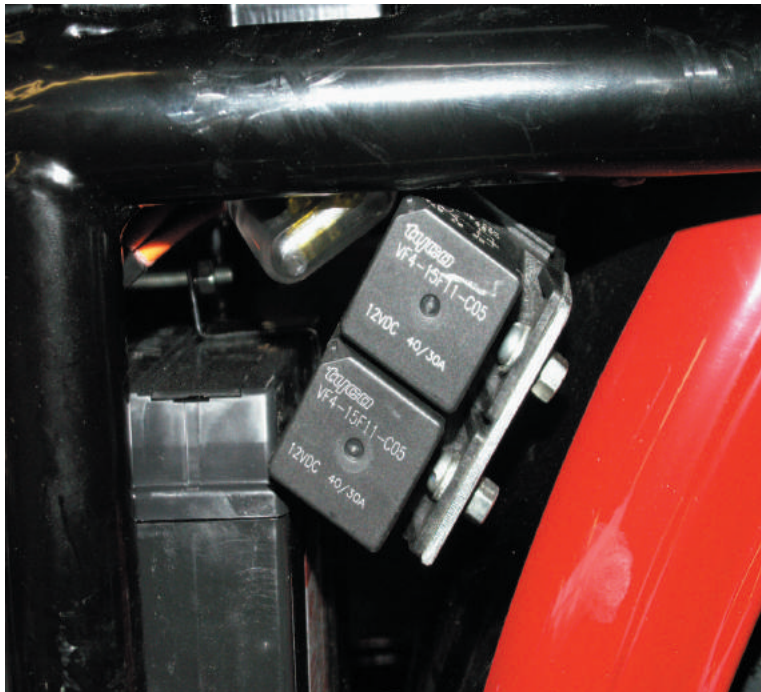
The headlight control relays # 1 & 2 are located underneath the fuel tank.
